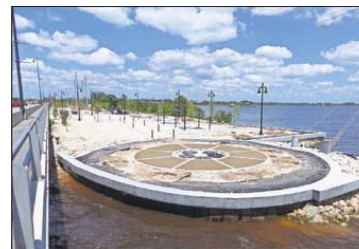
A much-improved seawall, constructed with sheet metal and rip-rap, is just one aspect of the Gateway Harbor Walk, which eventually will connect the east side of the northbound U.S. 41 bridge to Bayshore Live Oak Park.
